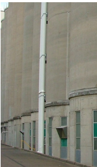
Silo 1212 & In-load pipes
